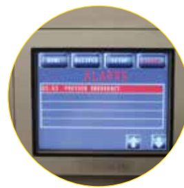
ALARMS INDICATING ERRORS
