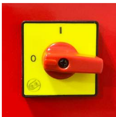
Switch set to "O" / "OFF": OFF or "disconnected", electric equipment sectioned from the electric feeding
